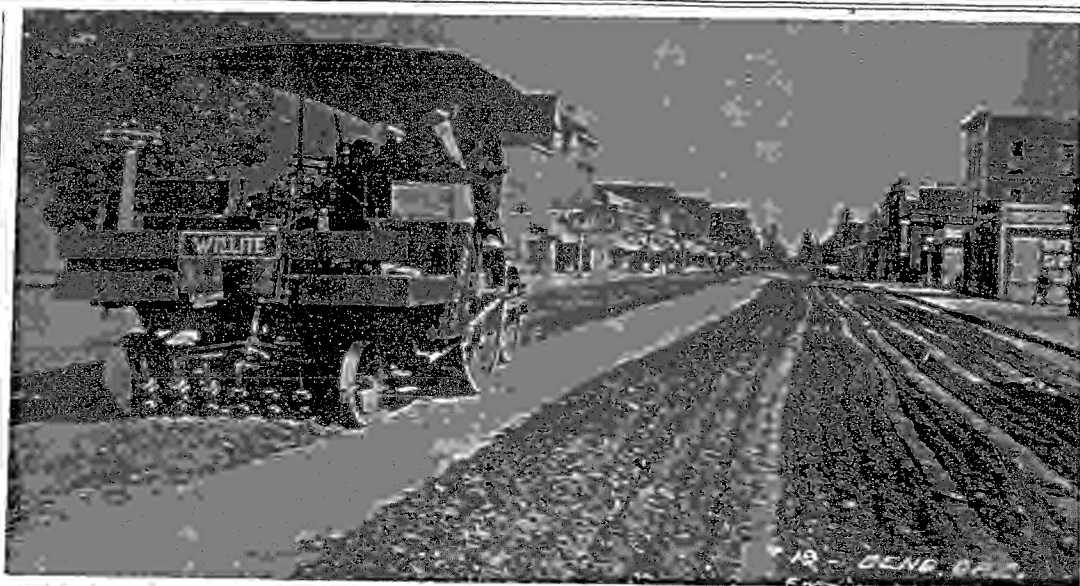
What's this? Plowing up Wall Street? The guess is correct, with the street being plowed, apparently in 1921, prior to the application of the controversial Willite pavement. The surface cracked and went to pieces in a few years. The view in this picture is to
